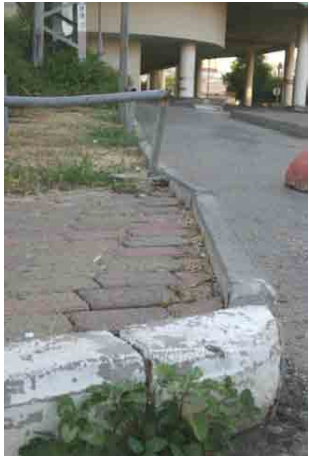
Fig 8. Pavement on the western entrance to Lev-Hamifratz shopping center parking.
